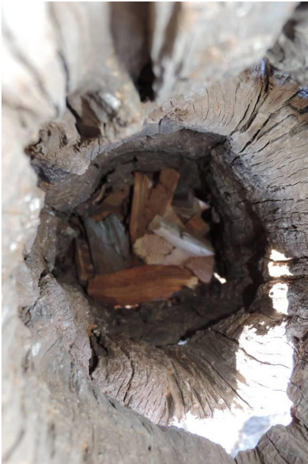
Figure 29. Blocks (or coarse chips) of Callitris can be placed inside the cavity to fill it to the desired level of the proposed cavity floor. These are best supported by a sub-floor of wire mesh tech screwed into place.
