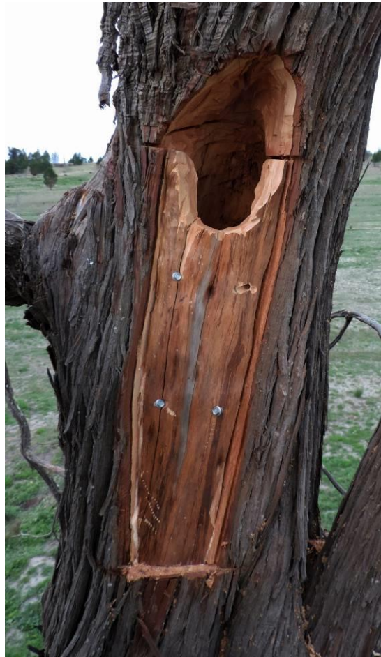
Figure 13. Replacement of the face plate should include some sealing of gaps between the trunk and the face plate. Long tech screws should be used to secure the face plate.
