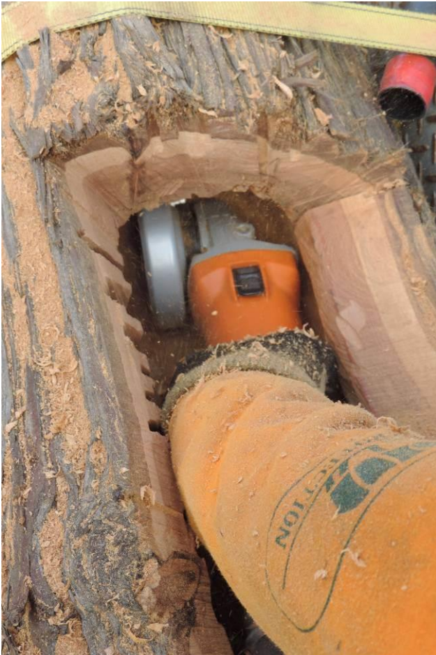
Figure 41. The large Arbortech blade being used to carve the inside of the cavity being worked. Note the red tip of a vacuum cleaner above the work area.
